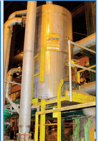
STAINLESS STEEL TANKS
